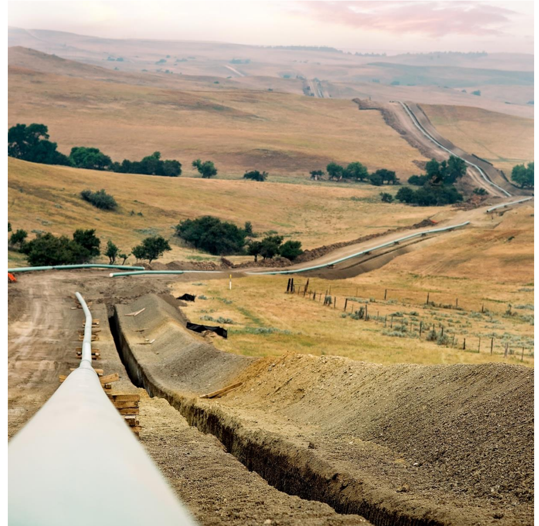
Note: Picture highlights 2021 installation of CCA CO 2 pipeline in Rocky Mountain region
